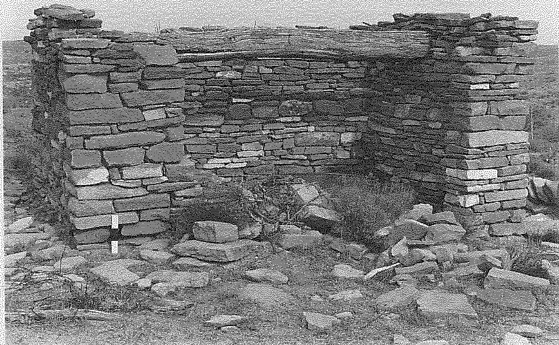
Figure 13. Rock outbuilding with large viga. Front wall has collapsed; doorway is on left; facing north.
