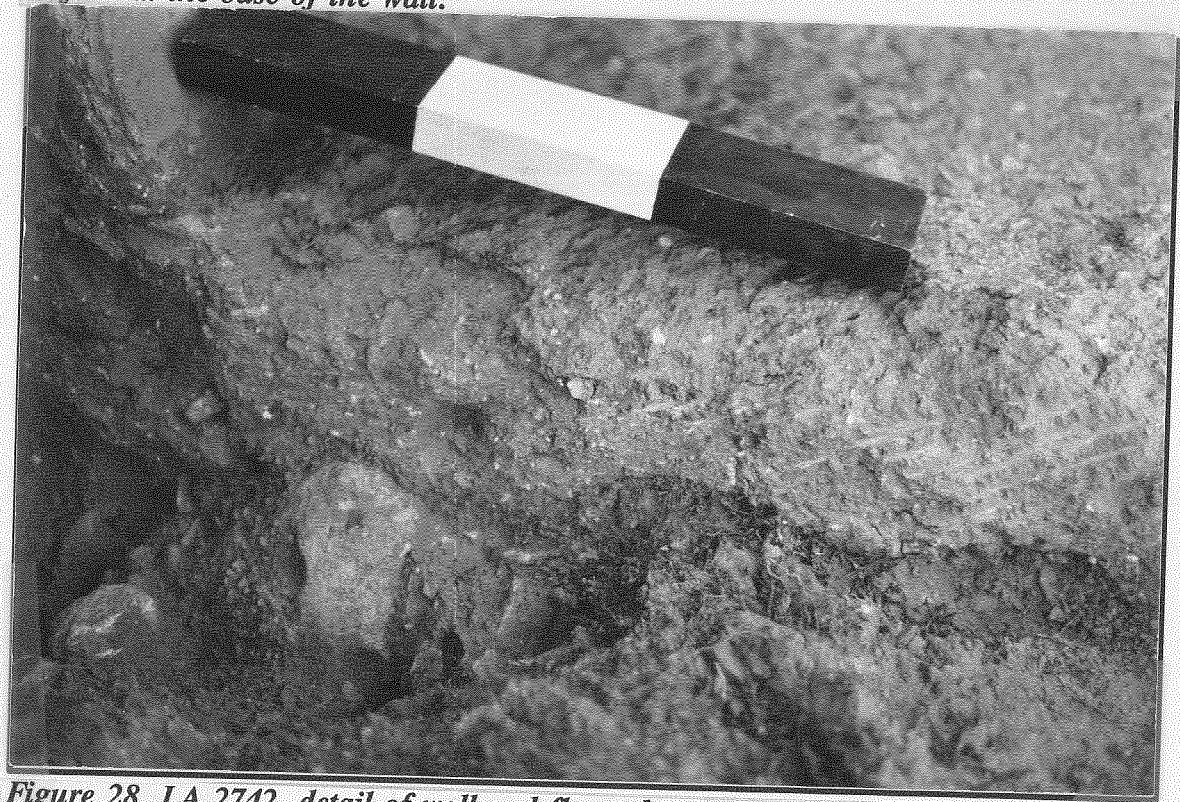
Figure 27. LA 2742, detail of wall and floor construction. Note the curved outer surface at the base of the wall.
