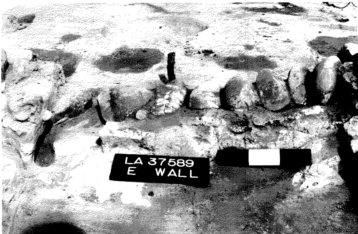
Figure 28. Foundation of the east wall of Room 1, LA 37589; cobbles have been placed in a shallow trench.
