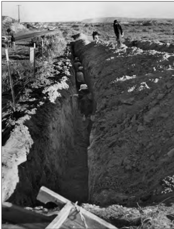
Figure 10.2. LA 37594, site setting, view north, along backhoe trench adjacent to existing right-of-way fence.
