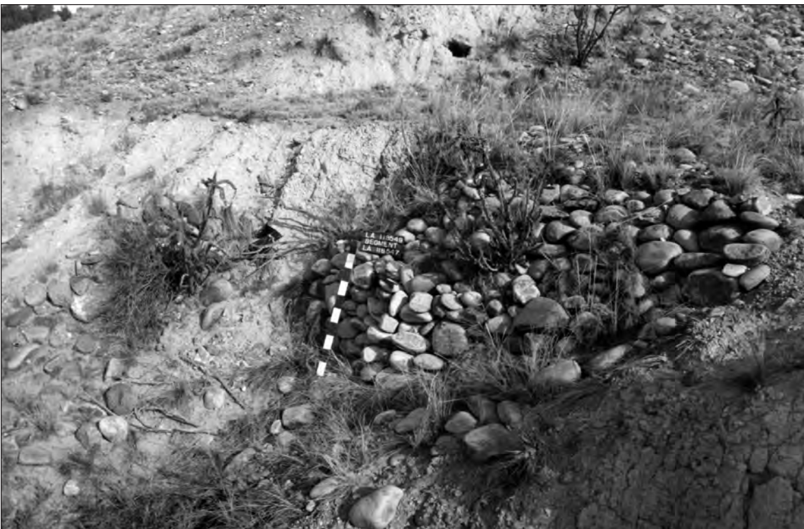
Figure 17.4. Probable historic retaining wall built with unmortared cobbles to partly block a drainage cutting through the trail, LA 118547.
