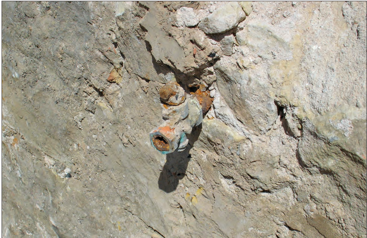
Figure 16.4. Water spigot installed in the east wall of Room 1, Structure 6.
