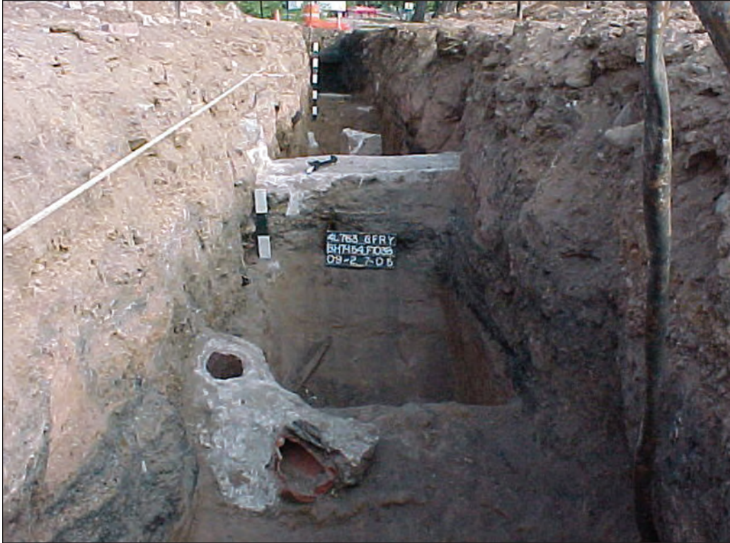
Figure 6.23. LA 149916, Feature 1038, from the south. A concrete pipe riser lies in the left foreground; a concrete wall foundation crosses through the center; concrete piers extend down the trench.
