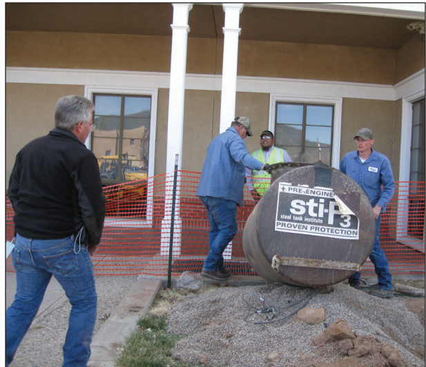
Figure A2.16. End of steel diesel tank and state inspectors, facing west.
