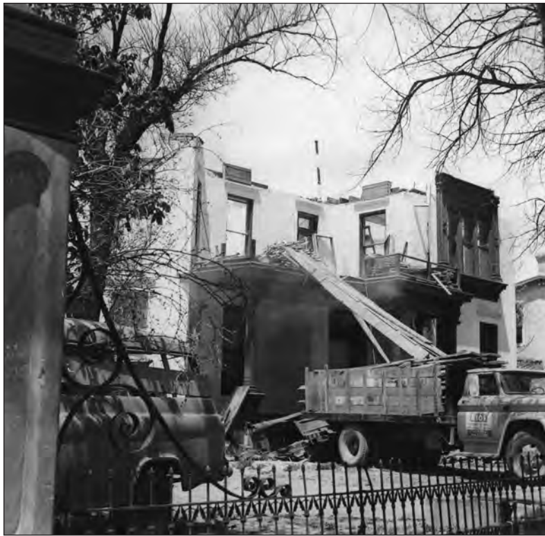
Figure 4.8. Dismantling of the Catron house on Grant Avenue, 1964, Santa Fe (courtesy Palace of the Governors Photo Archives, NMHM/DCA, neg. no. 029077).
