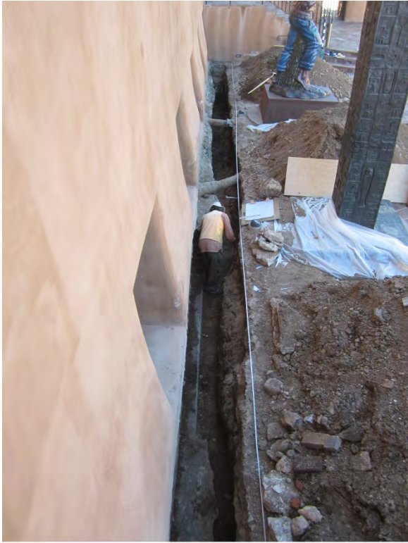
Figure 12. Monitoring trench, current project, along the museum's St. Francis Auditorium, view south.
