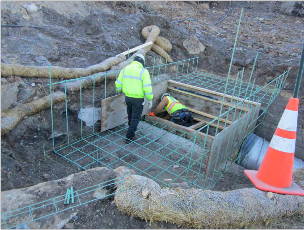
Figure 6.38. Rebar and wood forms are installed at the upper inlet of Feature 12, view southeast.
