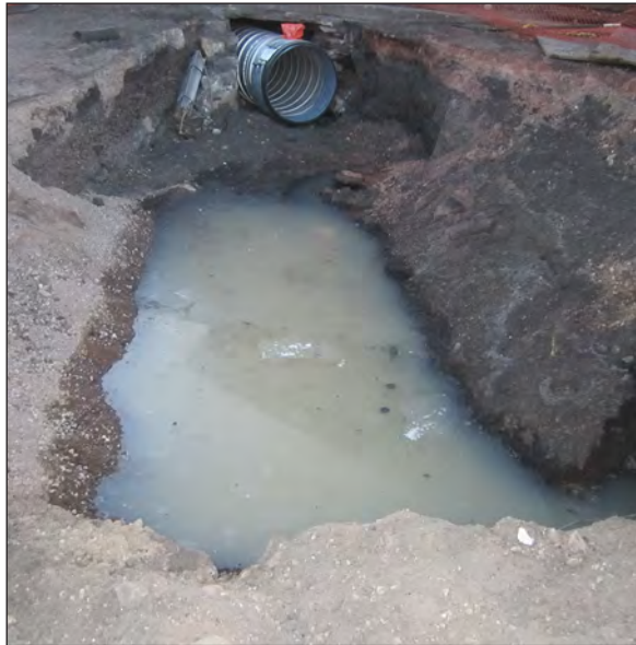
Figure 6.22. Broken sewage lines, view northeast.
