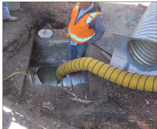
Figure 6.37. Oxygen is pumped to crew bolting slip liner to box culvert, view north.
