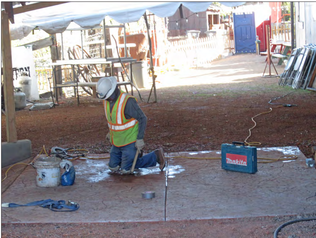
Figure 6.78. AUI crew member stamps a design into the uncured concrete pad, view north.
