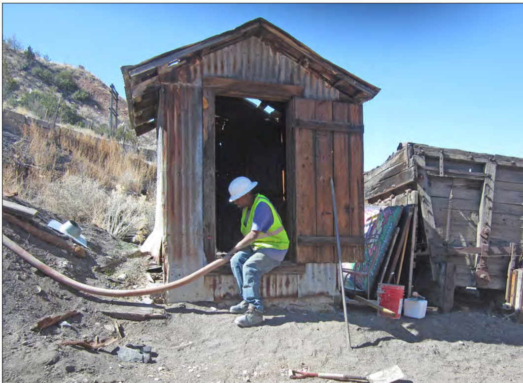
Figure 6.66. Con Deck crew member pumps grout below pump house into Feature 12 box culvert, view southwest.
