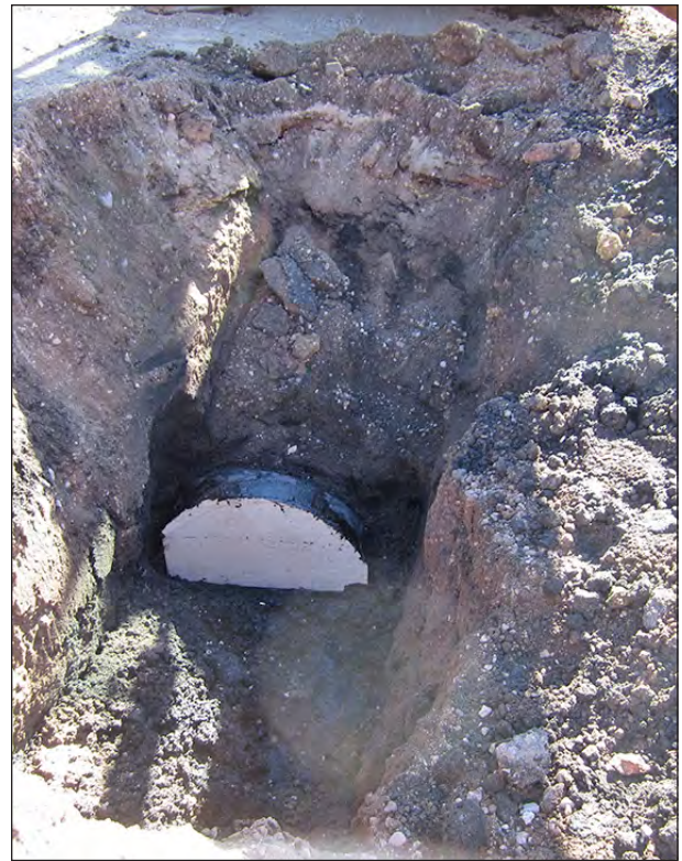
Figure 6.73. Plugged infiltrator, view east.
