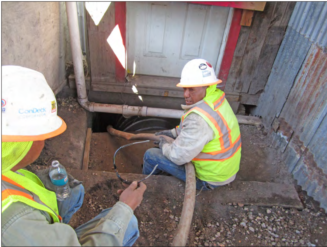
Figure 6.61. Con Deck crew pours grout into the Old West Saloon's drop inlet, view west.
