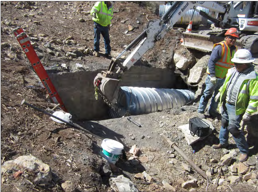
Figure 6.36. Sections of culvert are inserted through upper inlet of Feature 12, view south.
