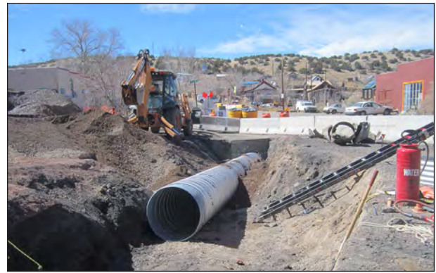
Figure 6.24. Slip liner connected to lower drop inlet at NM 14, view southwest.
