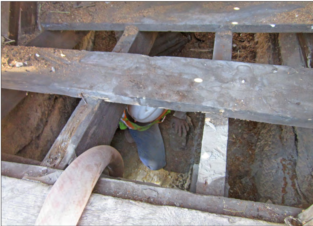
Figure 6.67. Con Deck crew member pumps grout below pump house into Feature 12 box culvert, view southwest.
