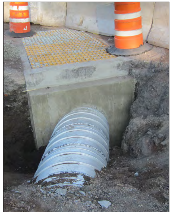
Figure 6.35. Slip liner in new concrete wall at lower drop inlet, view southwest.
