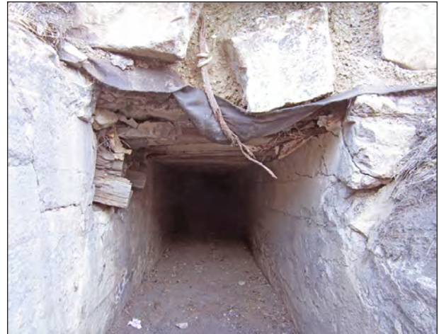
Figure 6.1. Opening to upper inlet of the historic concrete box culvert, view west.
