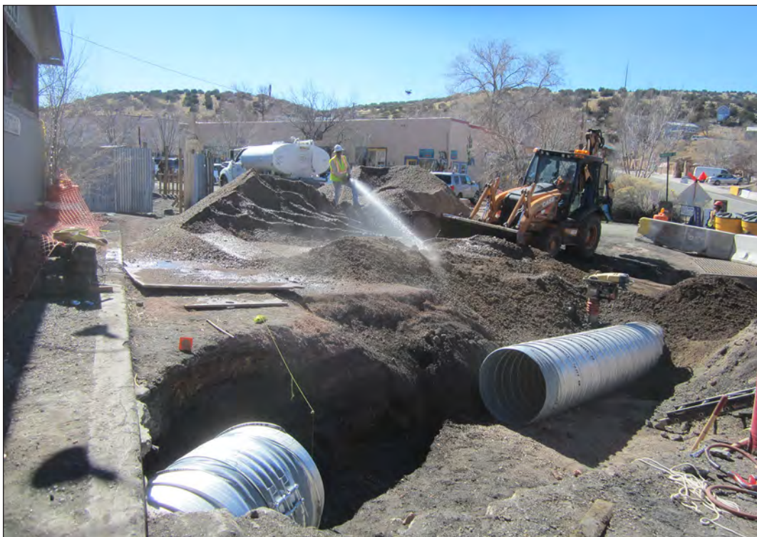
Figure 6.25. Base course is hosed down to cover the slip liner, view southwest.
