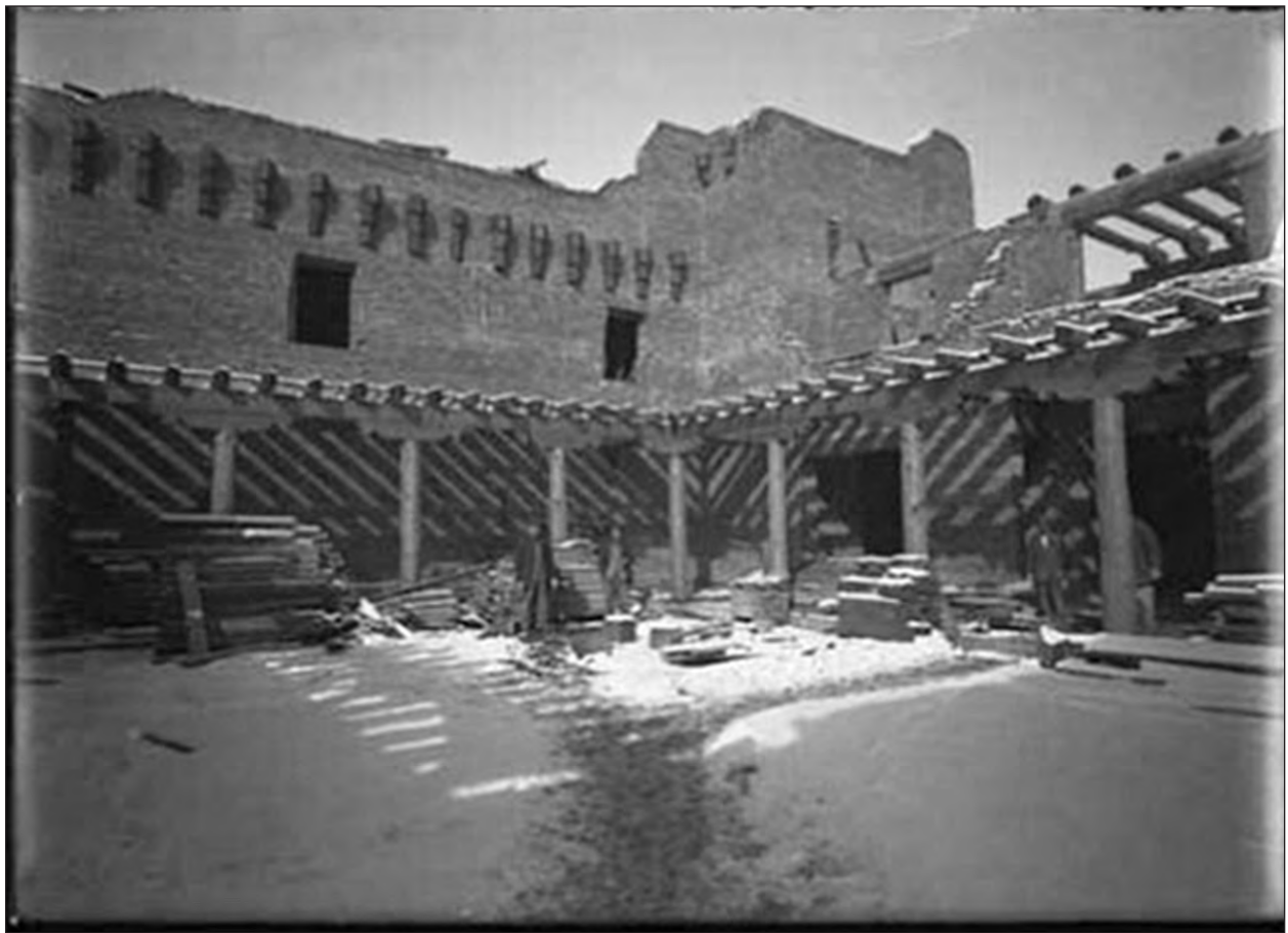
Figure 4. View of the northwest corner of the Museum of Art courtyard during construction in 1917.
