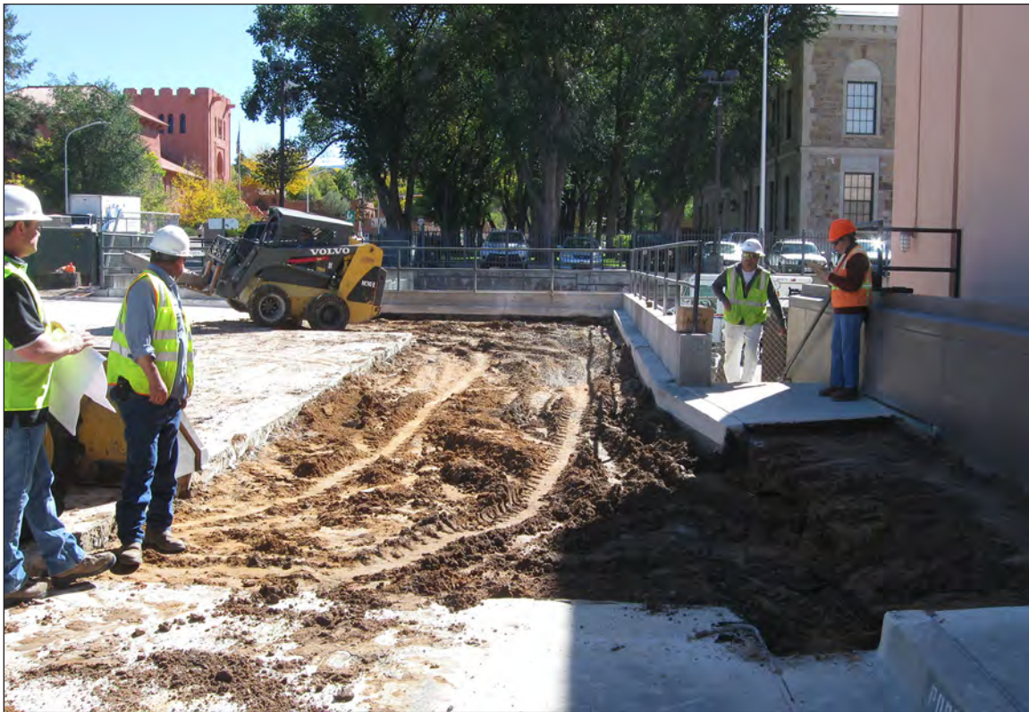
Figure 5.1. Excavation area after the removal of the concrete parking lot, view east.
