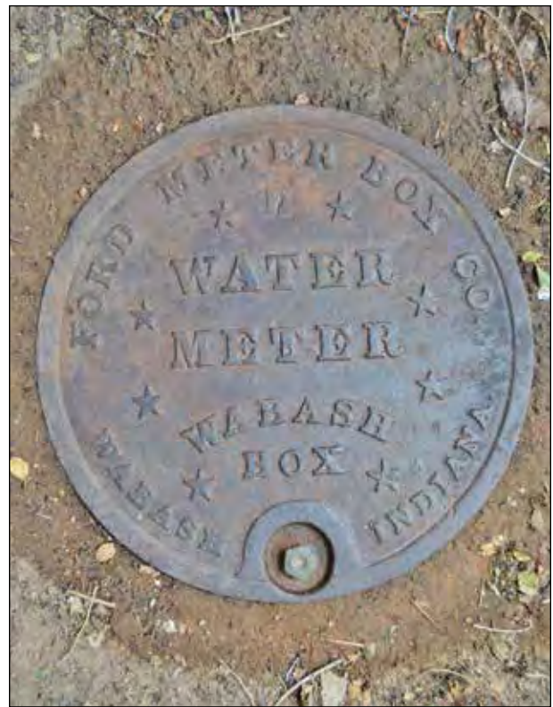
Figure 10.5. Ford Meter Box Company meter cover from Camino Don Miguel.
